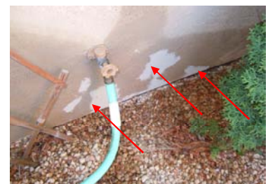
Surface damage to stucco color coat at north
