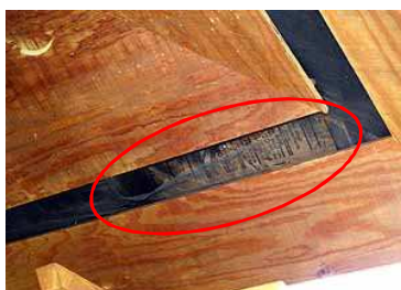
Soffit vent screen at NE corner was varmint damaged.
