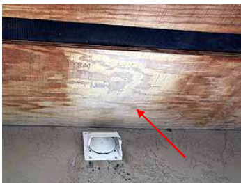
Bleached soffit finish at dryer vent
